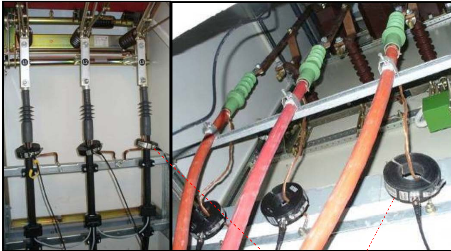
Fig. 3: HFCT sensor attachment inside of switchgear Sensors at Cable Mid-points
